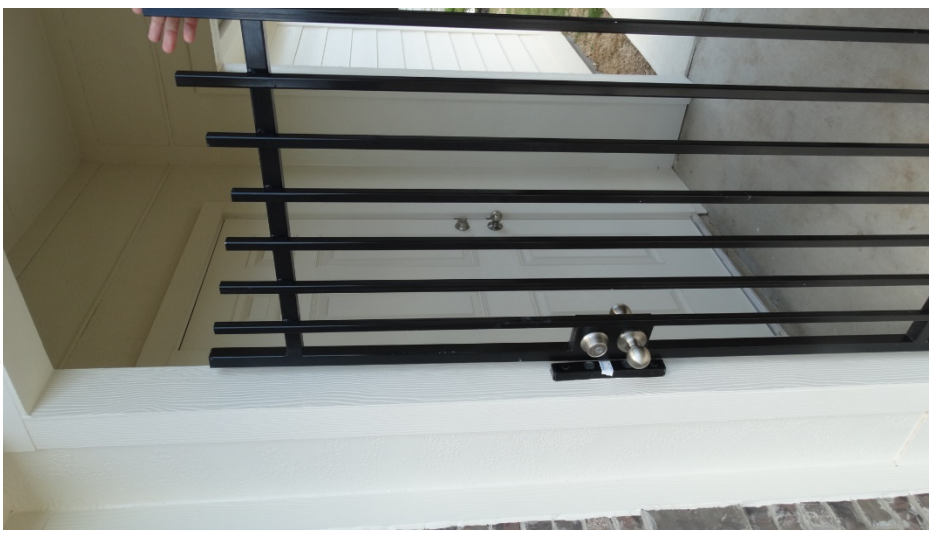
Entrance Gate — Deadbolt Lock
