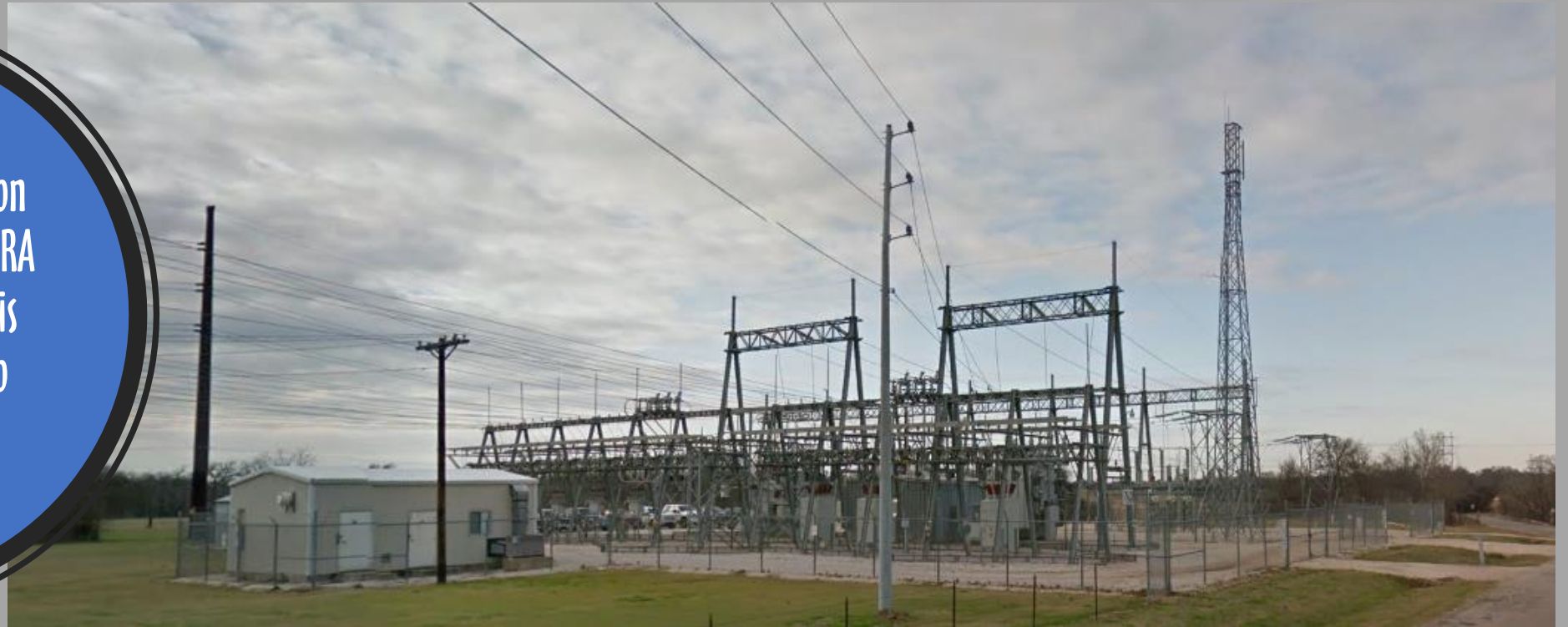
Main Street Sub-Station
